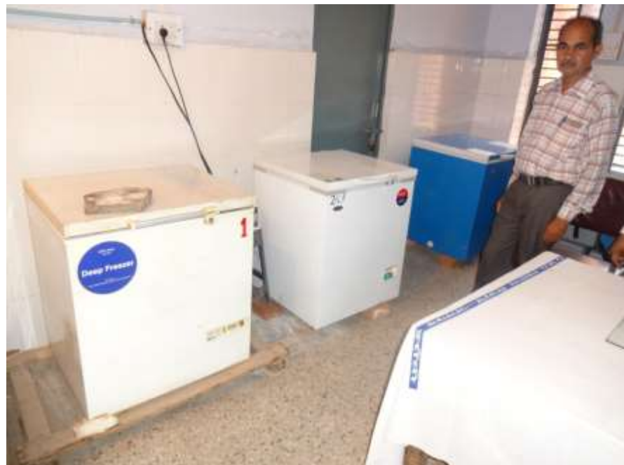
Figure 44: Cold chain equipment at CHC Mauranipur.
