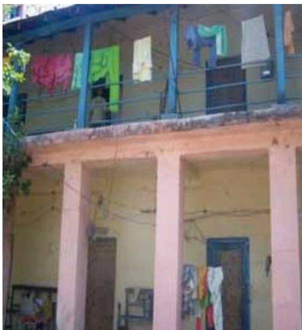
The hostel building allotted to staff nurses in Pauri Garhwal district hospital was in a condemned state with very scare water supply.
