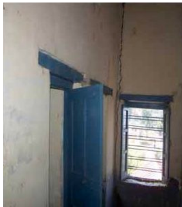
A large crevice inside the hostel building which may anytime fall apart.
